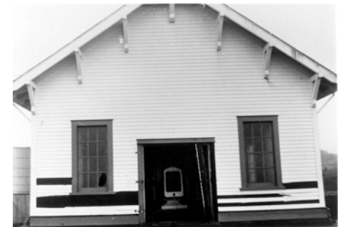
Damage to the west wall of the Fog Signal building following the storm.
